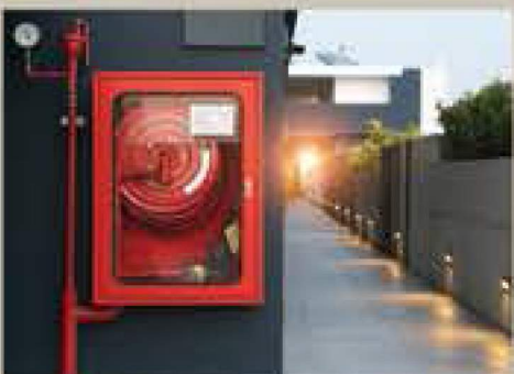
Fire Fighting System
