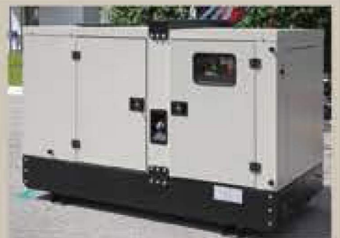
24x7 Power Backup
